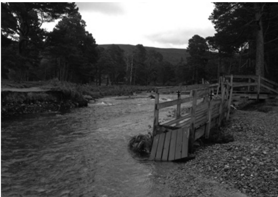
Footbridge over the Derry washed aside on the night of 10 th 11 th August
